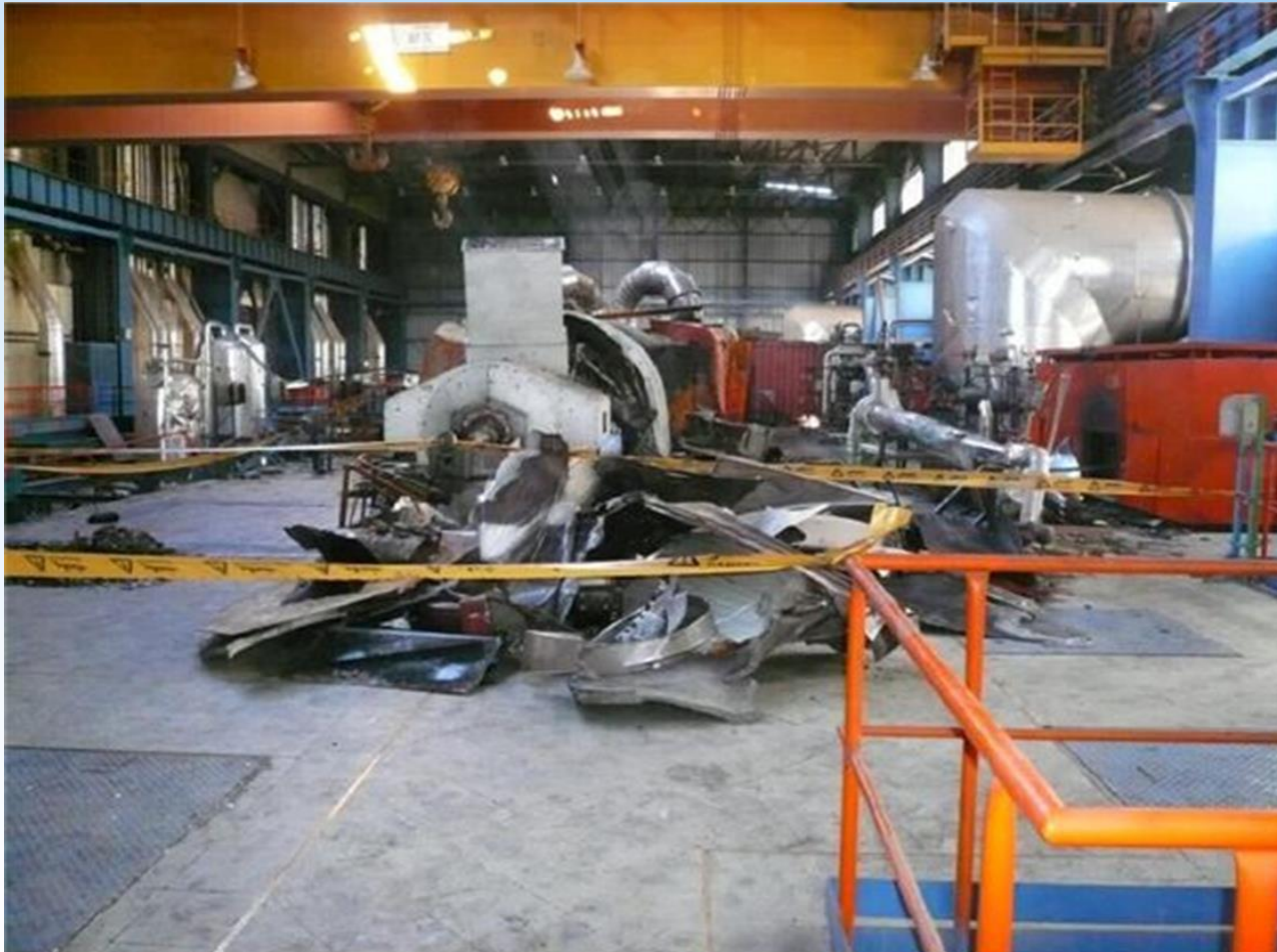
Iranshahr Power Plant Explosion- Coupling Failure
